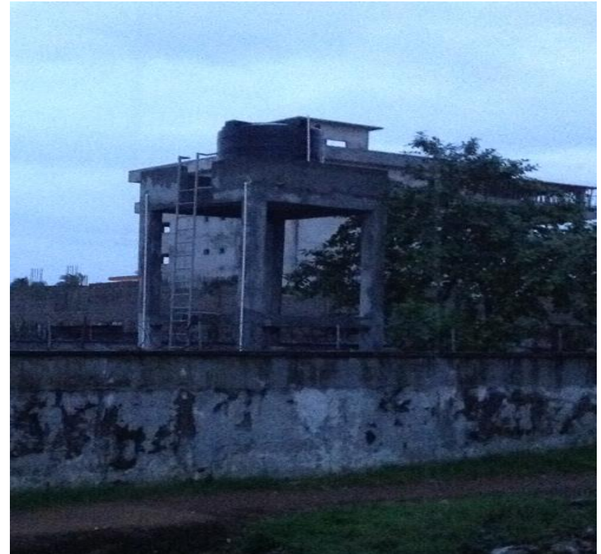
UNITED METHODIST WOMEN CONSTRUCTED A WATER TOWER TO PROVIDE CLEAN WATER FOR CHILDREN IN THE DAY CARE
